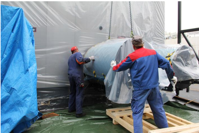
Figure 3 Installing a water cooled burner to the burner opening (outside of the boiler)
