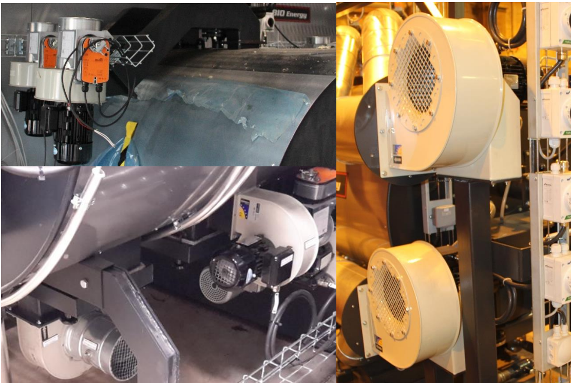
Figure 14. Burning air fan placement. On left, 1000 and 1500 kW on right.
