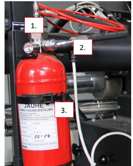
Figure 13. Powder fire extinguishing system installed on the feeder
