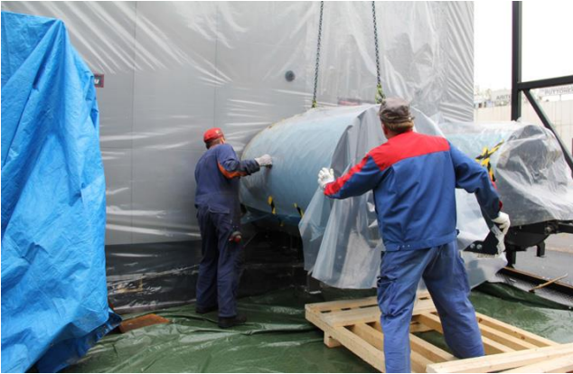
Figure 5. Fitting the burning compartment to the boiler's burner hole with a help of a lift.
